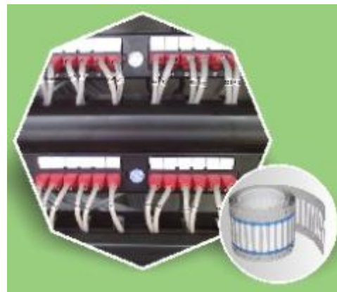
6. Identification Sleeve: permanent marking for Telecommunication cable.
